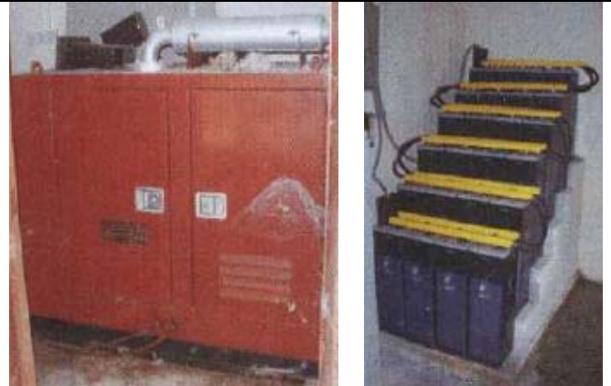
Genset and battery bank
