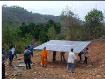
The solar PV system in the village
