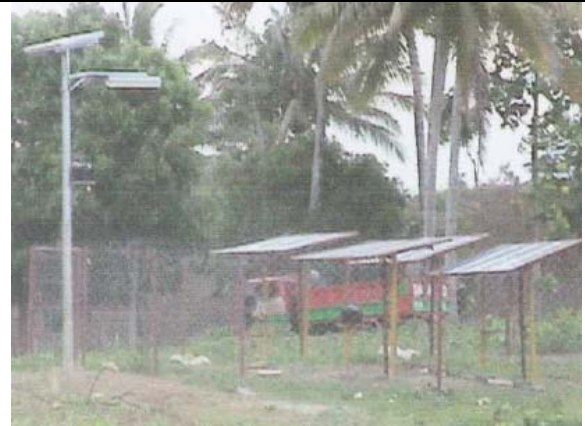
Solar street light and entire 4 channel solar battery charging station
