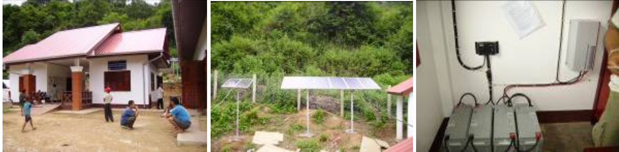
Ban Kuai health clinic and its PV system (Courtesy by Sunlabob Co.)
