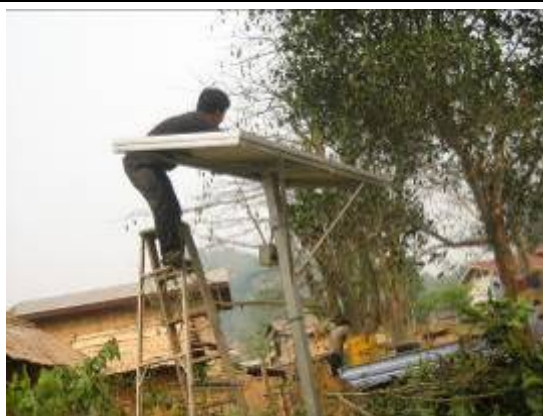
240 Wp PV array of battery charging station (Courtesy by Sunlabob Co.)
