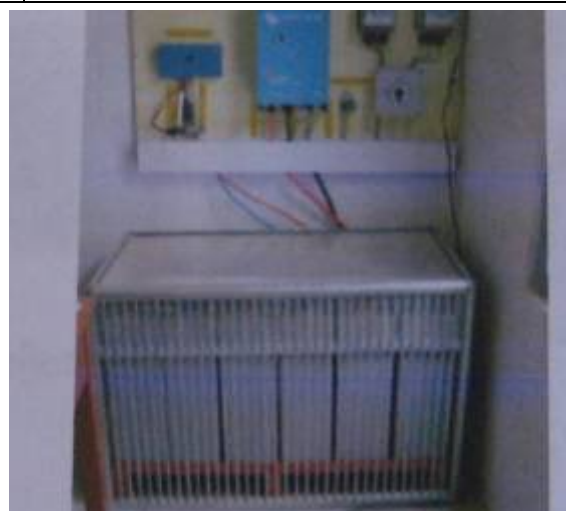
Batteries inside box and solar board above
