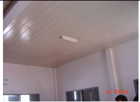
Figure 15: Lighting in the dormitory of the centre
