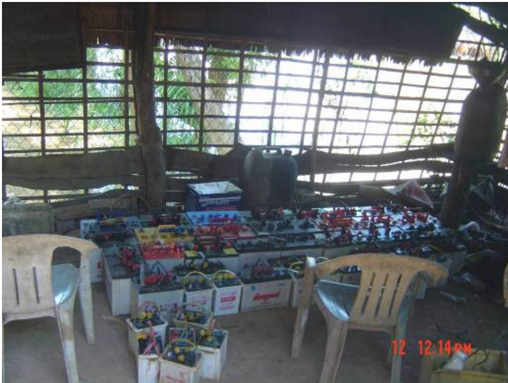
Figure 6: Battery Charging Station
