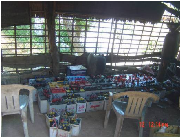
Figure 1: Battery Charging Station in Prek Chrey
